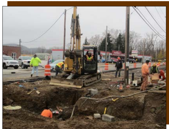
Scenes like this, sewer, water, energy, phone and road work, should end in mid-December if the weather holds and all goes well with the East State Street Reconstruction Project.
