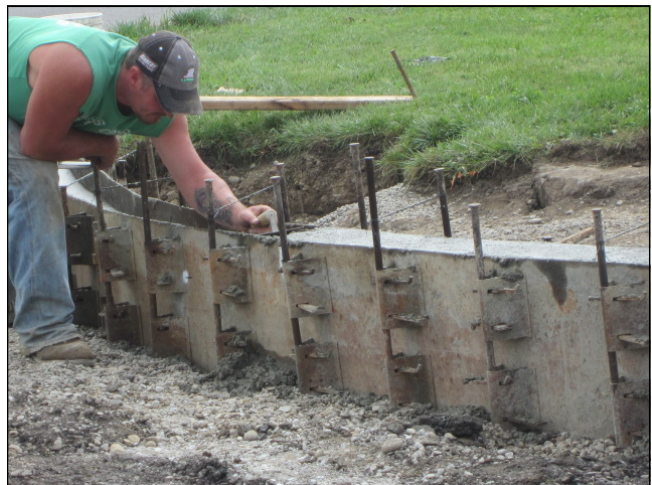
The hard-working crews have dressed up the landscape for a few months but will soon be a memory on East State Street. Officials are busy planning other projects to renew the city's aging infrastructure.
